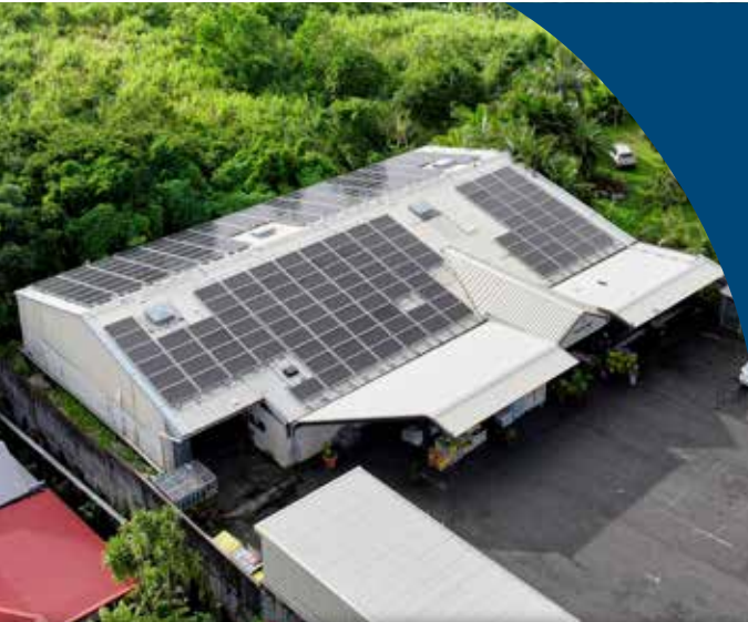
Rooftop installations on industrial and commercial buildings
